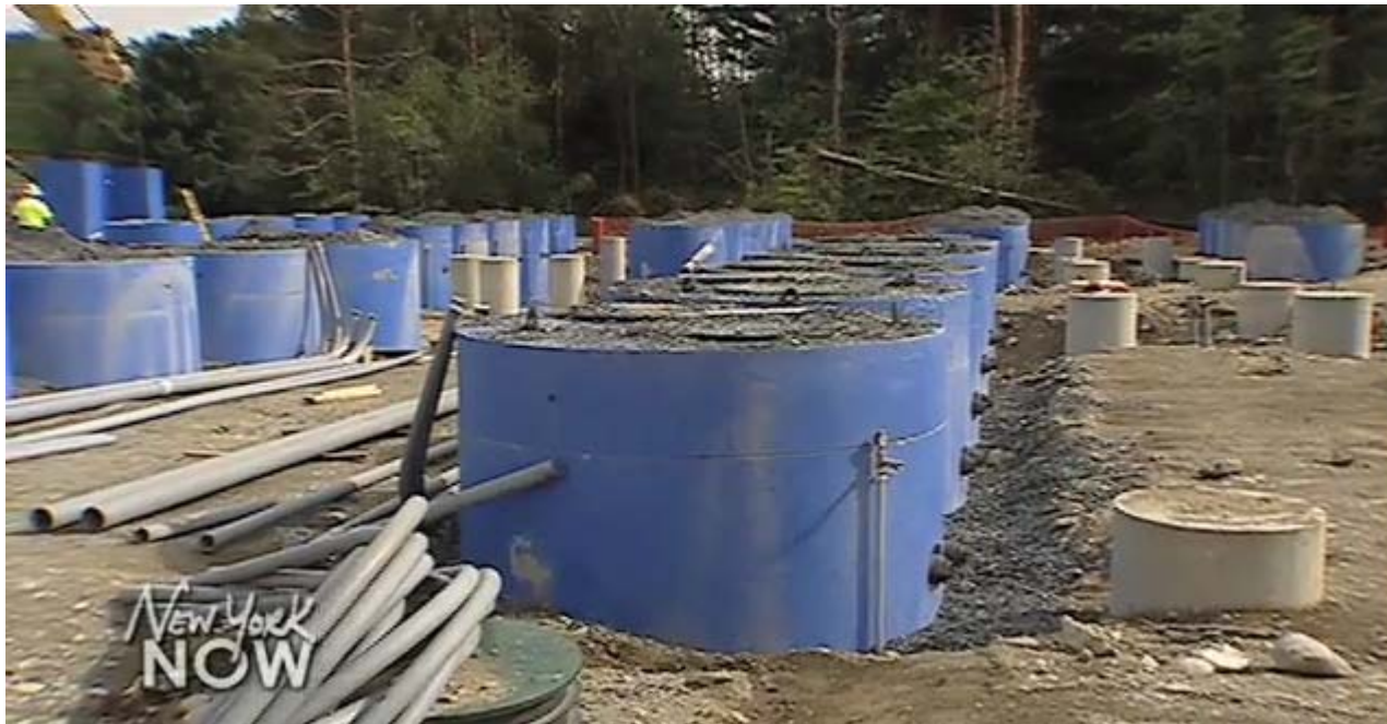
A Flywheel storage technology in New York by Beacon Power
